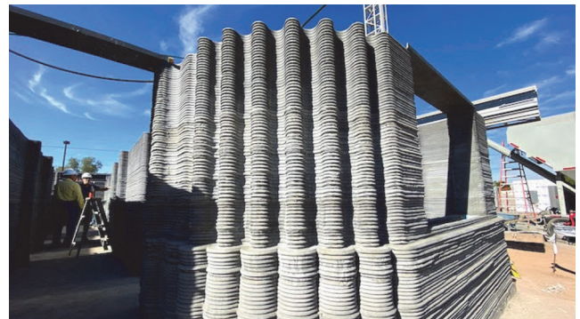
Figure 9. Three-dimensional printing of exterior and interior walls, left in their original layers [33]
